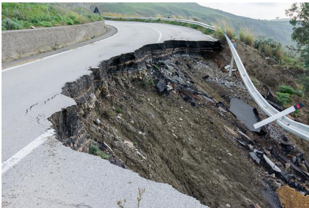
Geosynthetics can be used to improve drainage, mitigate erosion, and reinforce soils to prevent collapse.
