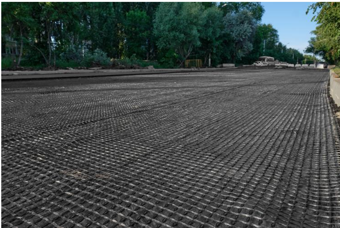
A geosynthetic interlayer installed ahead of the final asphalt layer. Geosynthetics are used in roadway bases and pavement systems to extend service lives and reduce maintenance.
